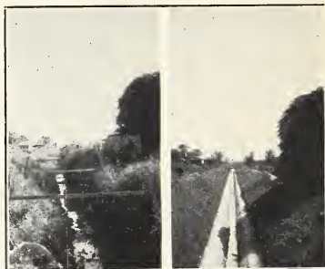
FIG. 5. Tunica, Mississippi. Left, before malarial control drainage; right, after construction of reinforced concrete invert with sodded banks.
